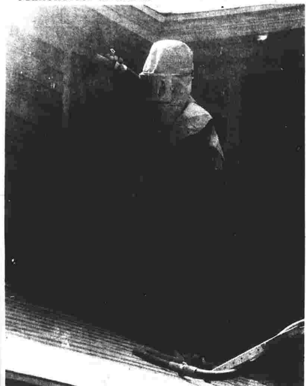
Evan Nay, working for Simsbury Sand Blasting, is surrounded by airborne particles as he sandblasts the exterior of a house at 182 Vernon St. The one-day job was done last week.
